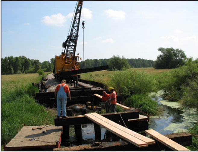
WSOR crews conduct superstructure repairs to bridge at Orfordville, WI to meet 286,000 pound industry standards.
